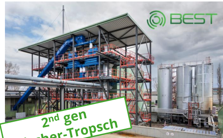
1 MW Syngas Platform Vienna
