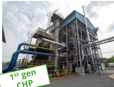
3.8 MW Nong Bua (Thailand)
